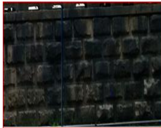
B) Algae colony on external wall surface
