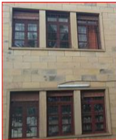
A). Deteriorated window of the building
