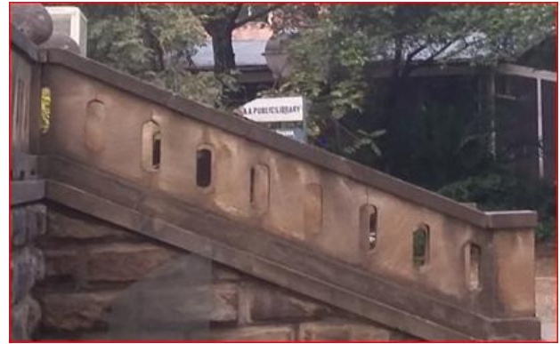
B) Deteriorated guard wall
