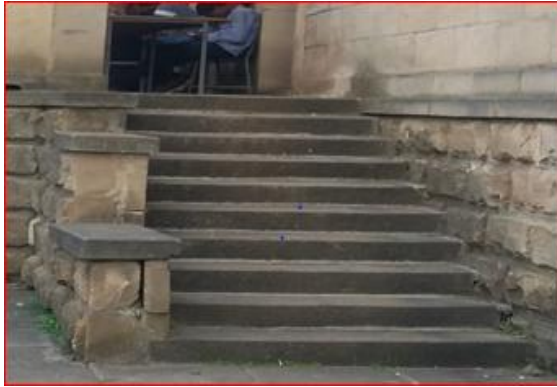
A) Deteriorated Steps of the building
