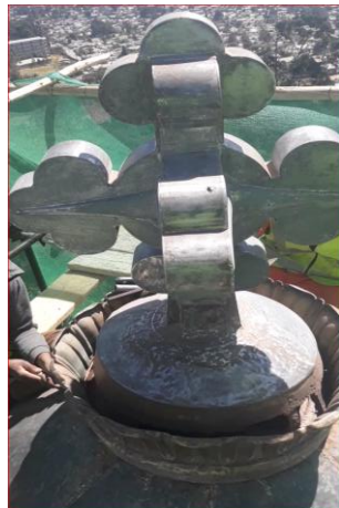
A) Deteriorated cross surface
