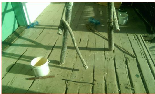
A) Deteriorated floor finish
