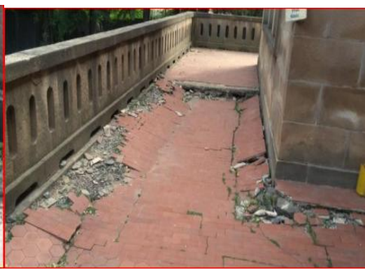
B) damaged tiles, floor finish on verandas
