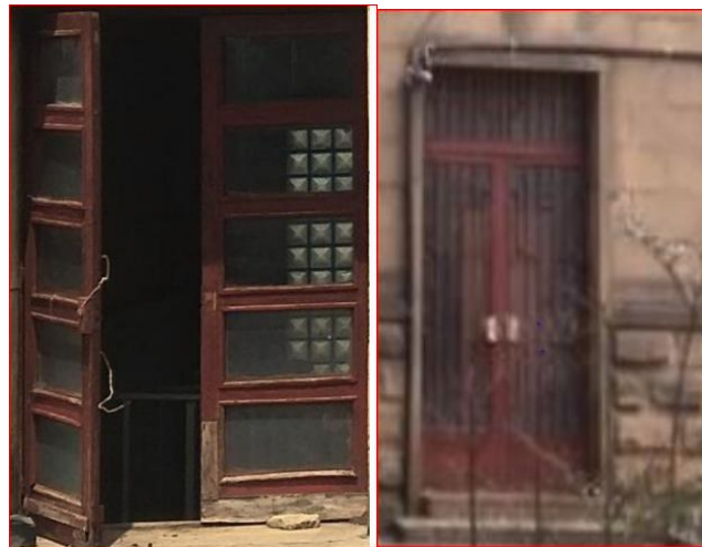
B) Deteriorated doors of the building
