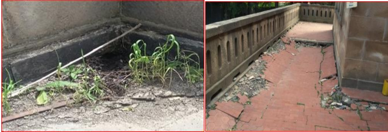
A) Growth of plants on the roof slab
