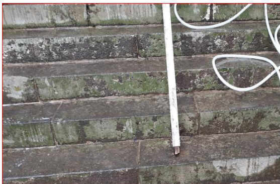
A) Algae and fungi colony on external staircase
