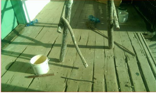
A) Deteriorated floor finish
