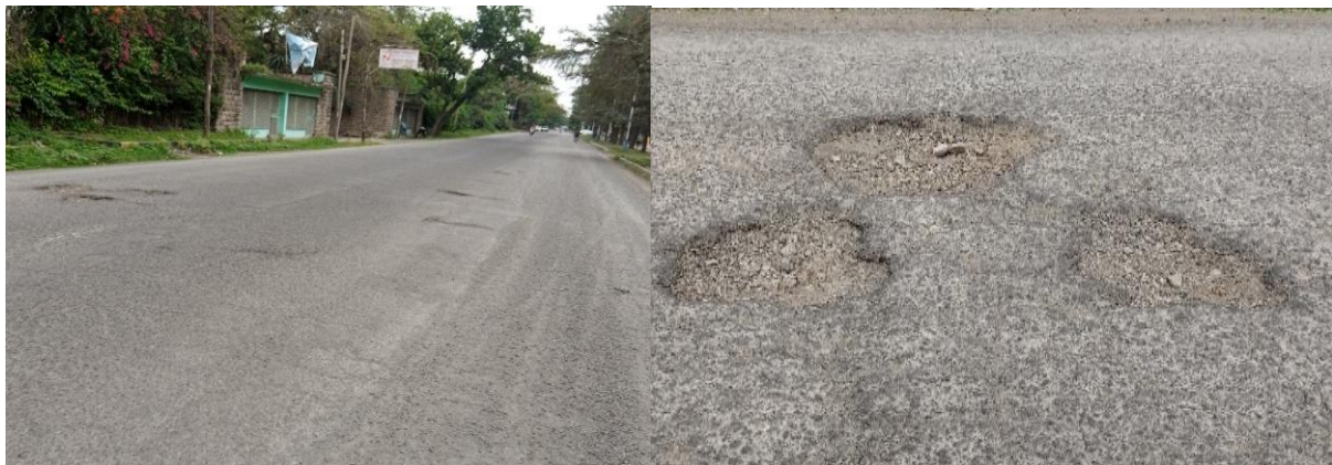
Figure 8. (a) Raveling (b) Pathole
