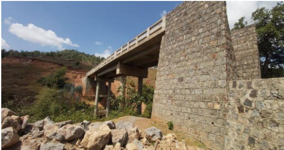
Figure 2. Partial View of Logita Bridge, abutment and approach embankment retaining wall under construction
